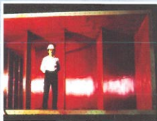
Exhaust Duct exit of Reverberant
